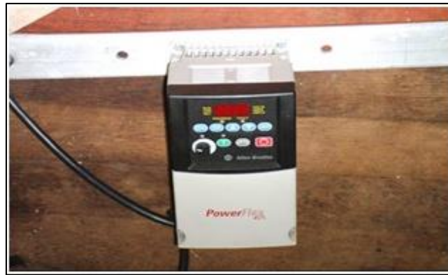
Fig 5: Shows the power supply to heat injection fan
