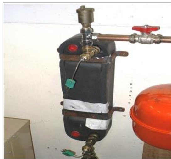
Fig 2: Shows the heat exchanger
