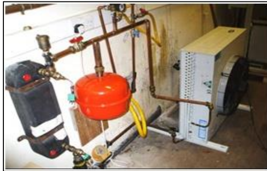
Fig 3: Shows the connections of the heat exchanger, water pump, heat rejection fan and expansion valve
