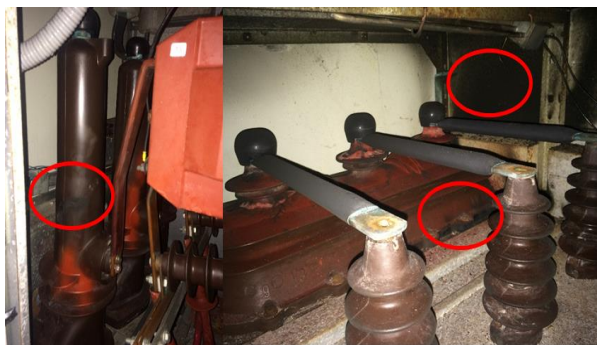
Figure 1: Flashover causing damage to Disconnect Switch and Load Balancing Switch as indicated by red circle. The picture was taken from the 20 kV cubicle at Lokomboro Micro Hydro Power Plant in Sumba, Indonesia (Photo by: The Author)
