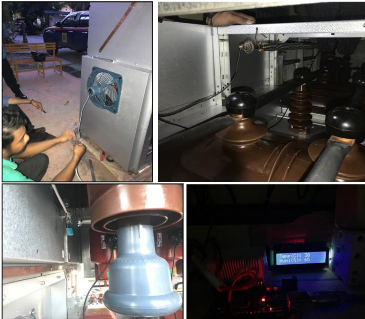
Figure 5: Installation of humidity and temperature control system component such as fan blower, heater, DHT11 sensor and LCD display (Photo by: The Author)
