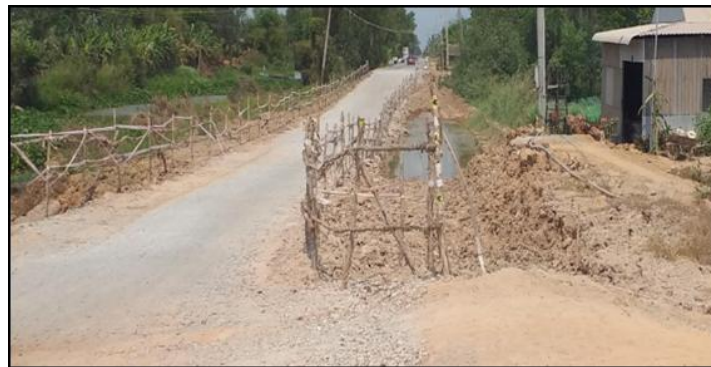
Fig-7: Overall segment of instability
